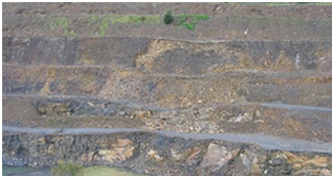
Figure 1: quarry slope failure
