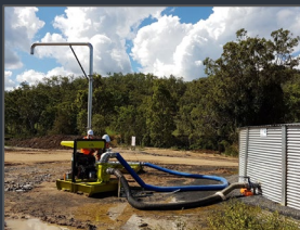
Diesel standpipe unit for fast water truck re-filling (Allflo)
