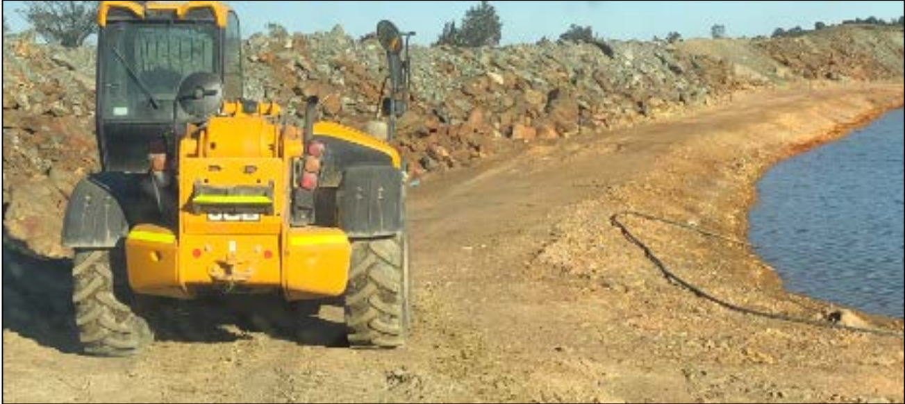
Figure 2 An example of an access road with an open edge, with insufficient controls in place to protect workers from exposure of driving into the open body of water.
